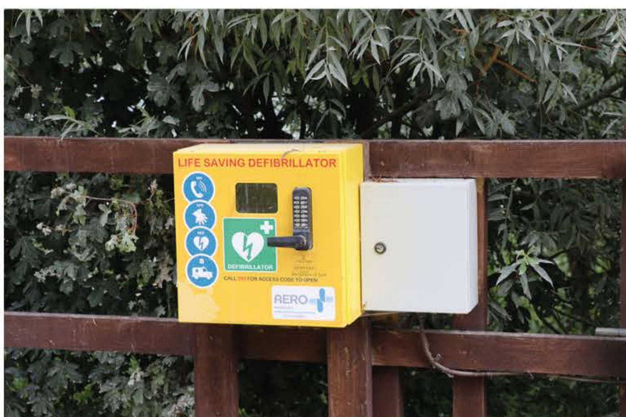
We now have six defibs on site.
